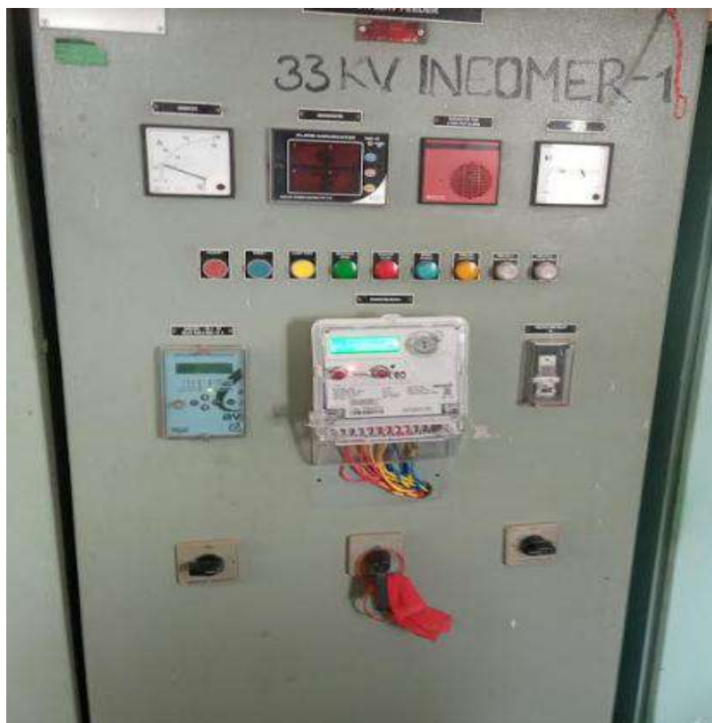
Control Panel of the substation
