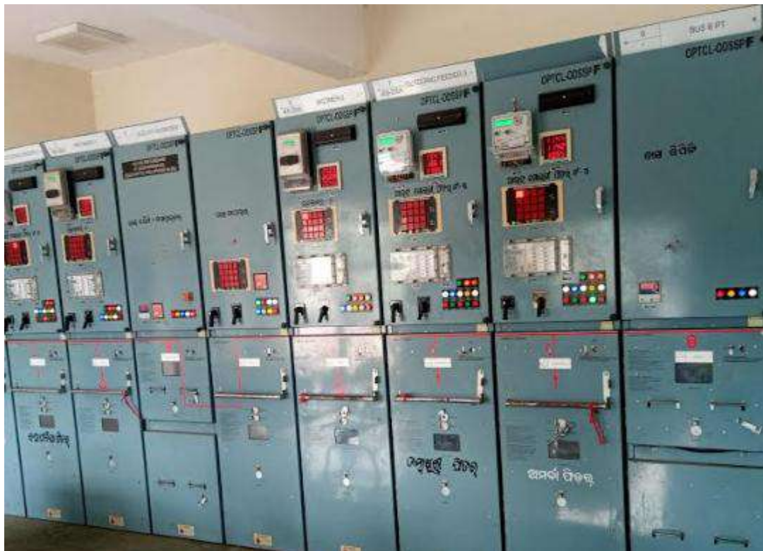
Control Panels at the Sub-Station.
