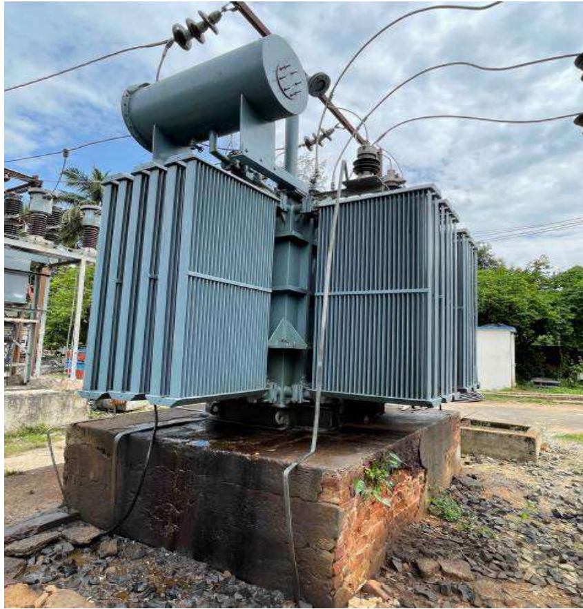
Oil Leakage issue of the Transformer at Nilgiri PSS.
