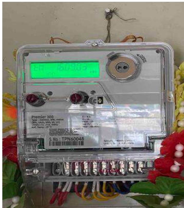
33 kV Incoming smart meter at the PSS
