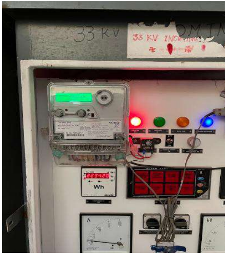
33 kV Incoming Smart Meter is in working condition
