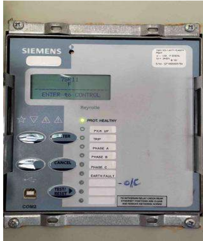
SCADA system implemented at the PSS.
