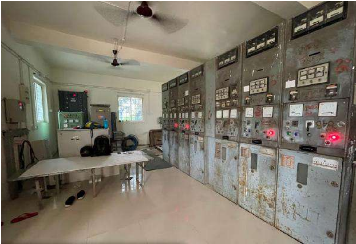
Control Panels at the 33/11 kV Gopalgaon Feeder.
