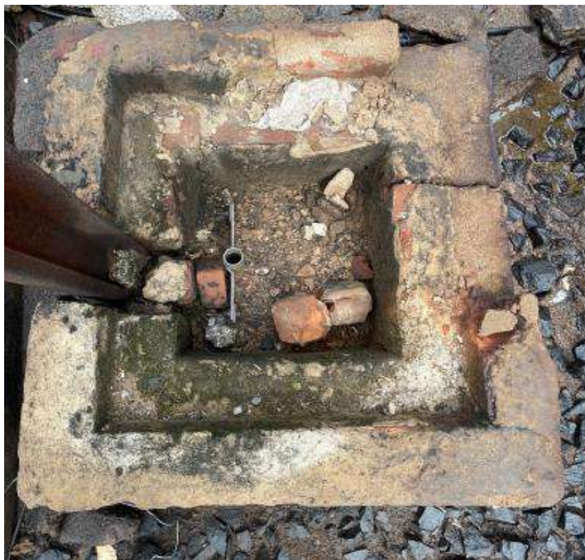
Earthing at the PSS
