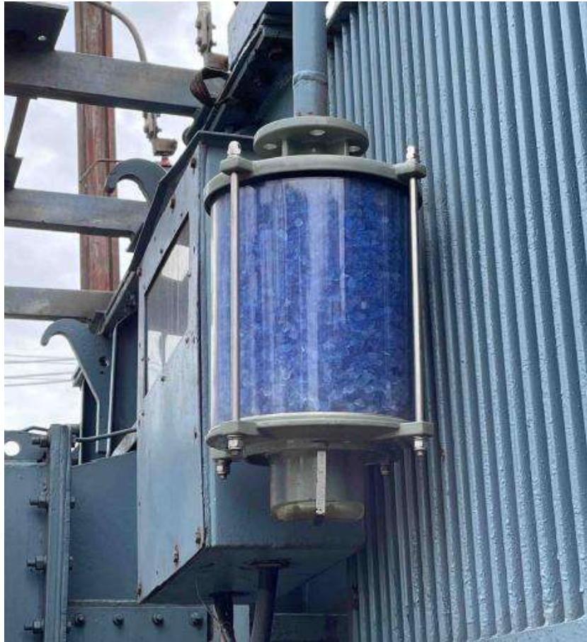
Silica gel of the Transformer is in good condition
