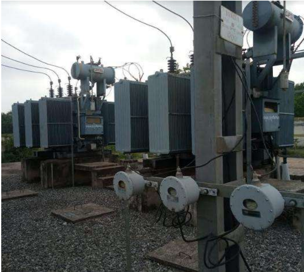
Power Transformers at the Sub-Station
