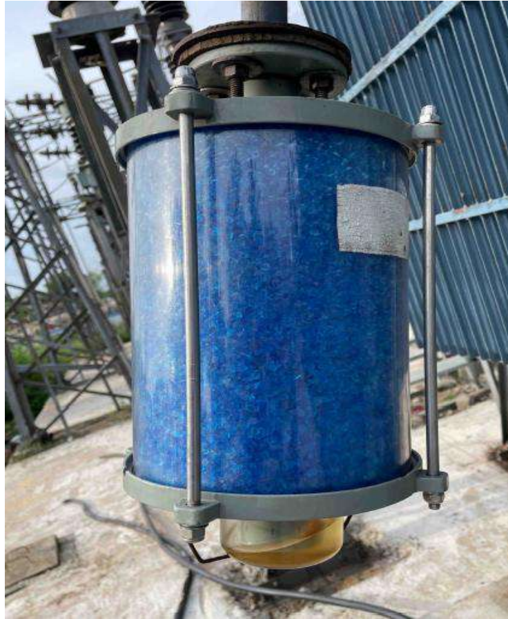
Silica Gel of Transformer at the PSS
