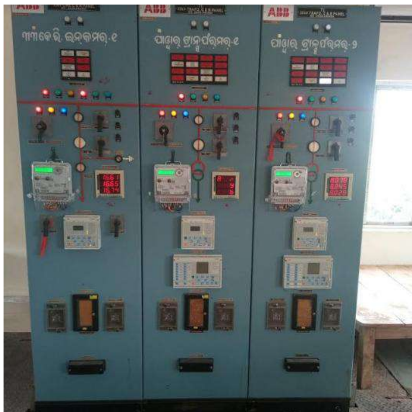
Control Panels at the Sub-Station.
