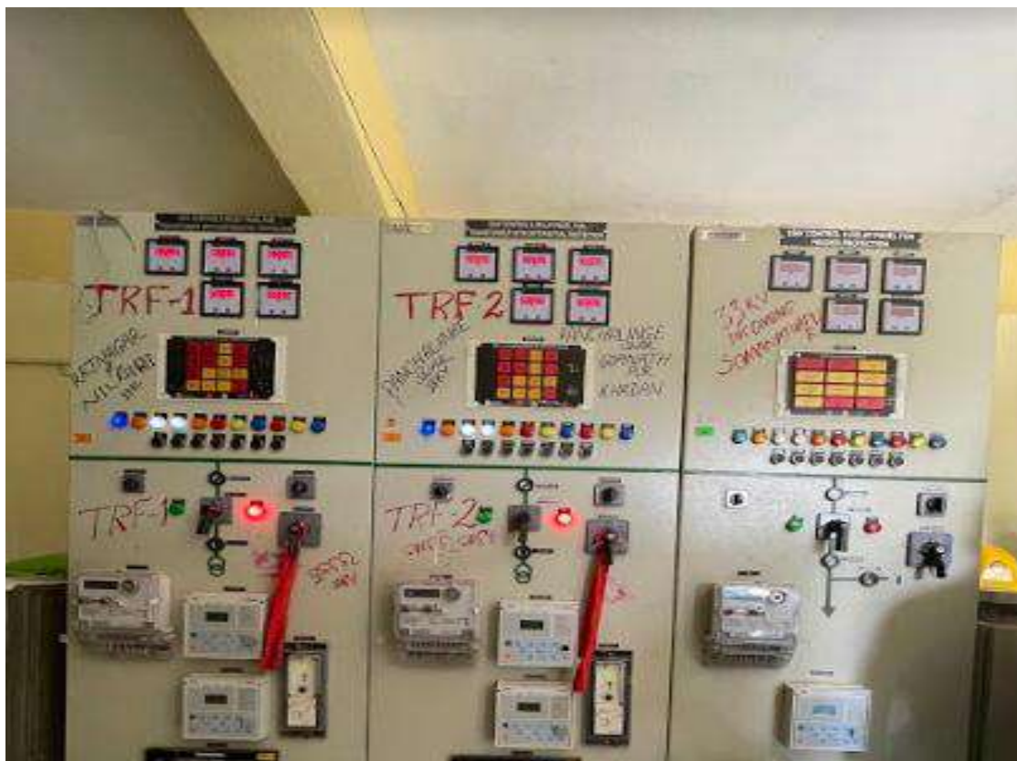
Control Panels at Nilgiri PSS
