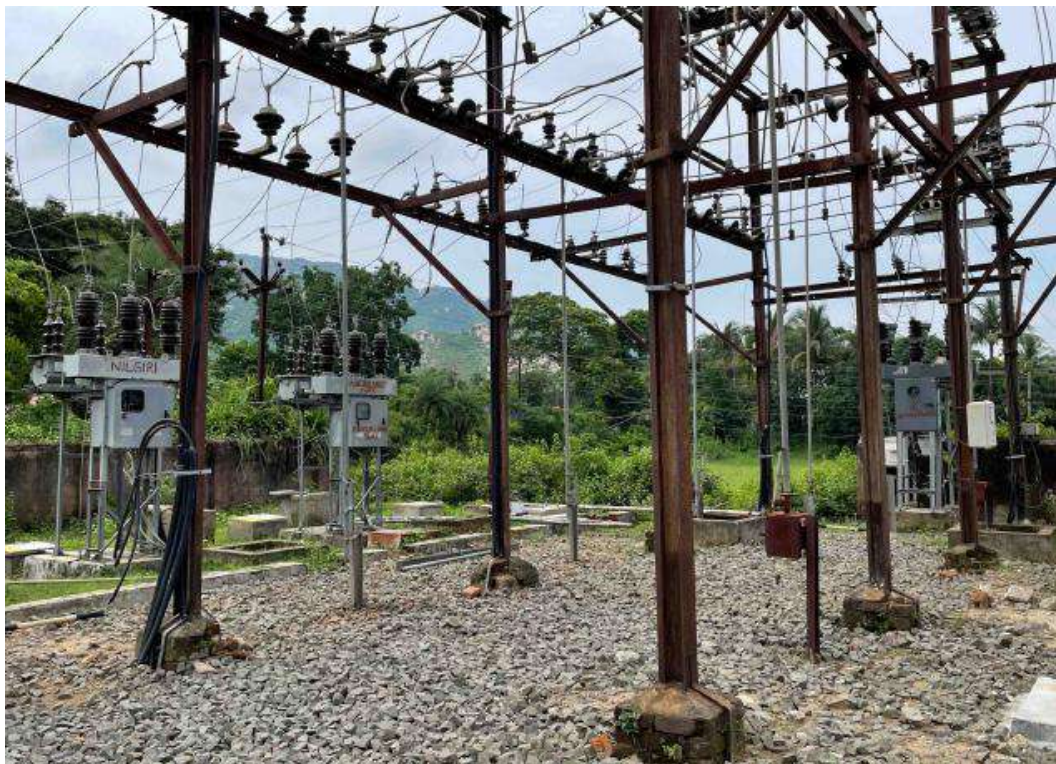
Broken boundary wall of the PSS
