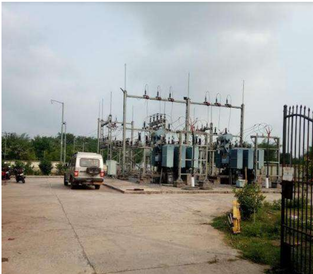
Visit to Gaon Armada 33/11 Kv Substation
