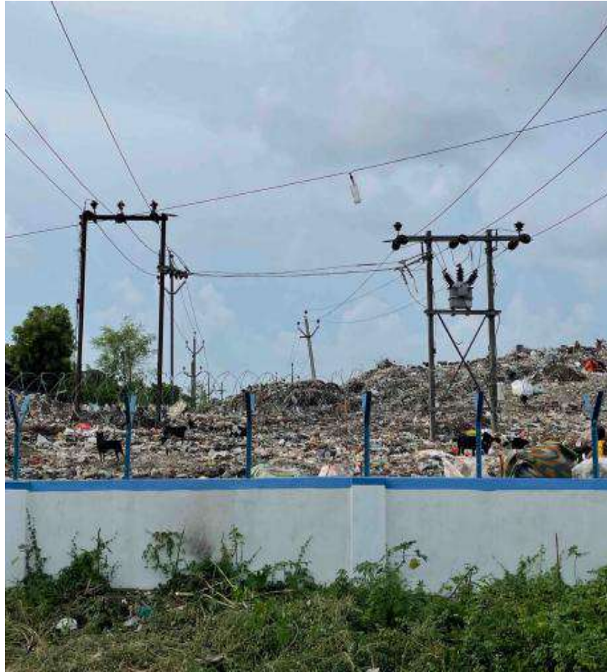
33kV Incoming line is very close to the ground causing safety issue
