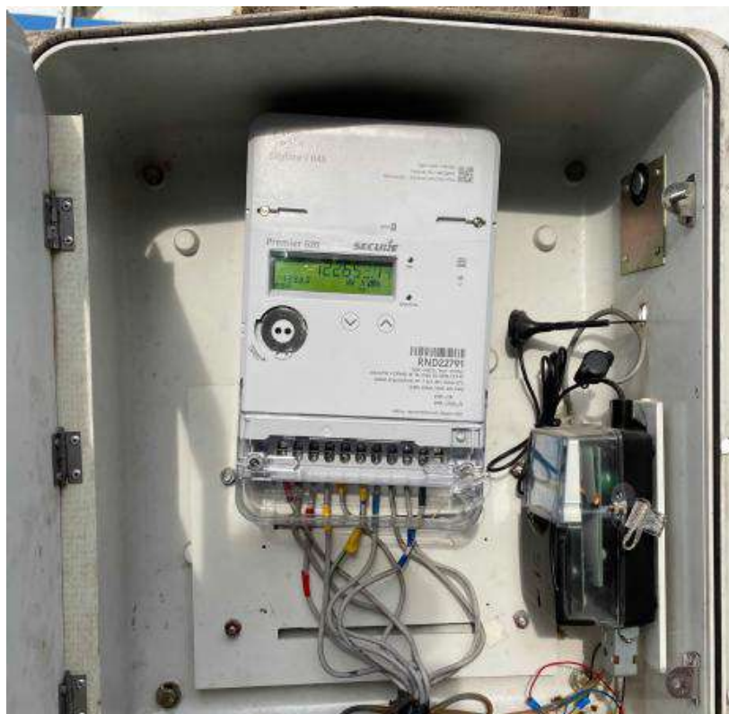
33 kV Incoming Smart Meter at the PSS
