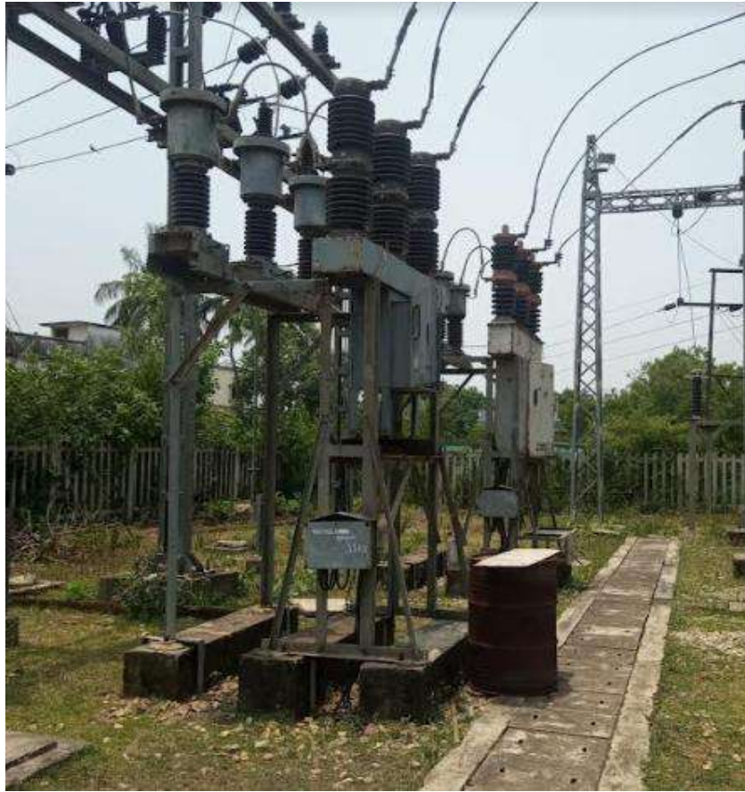
Manual VCB tripping at the substation
