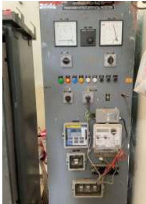
11 kV Control Panel
