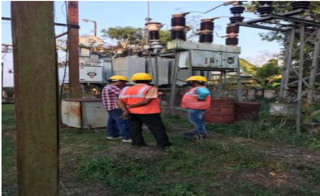
Visit to 33/11 kV PSS
