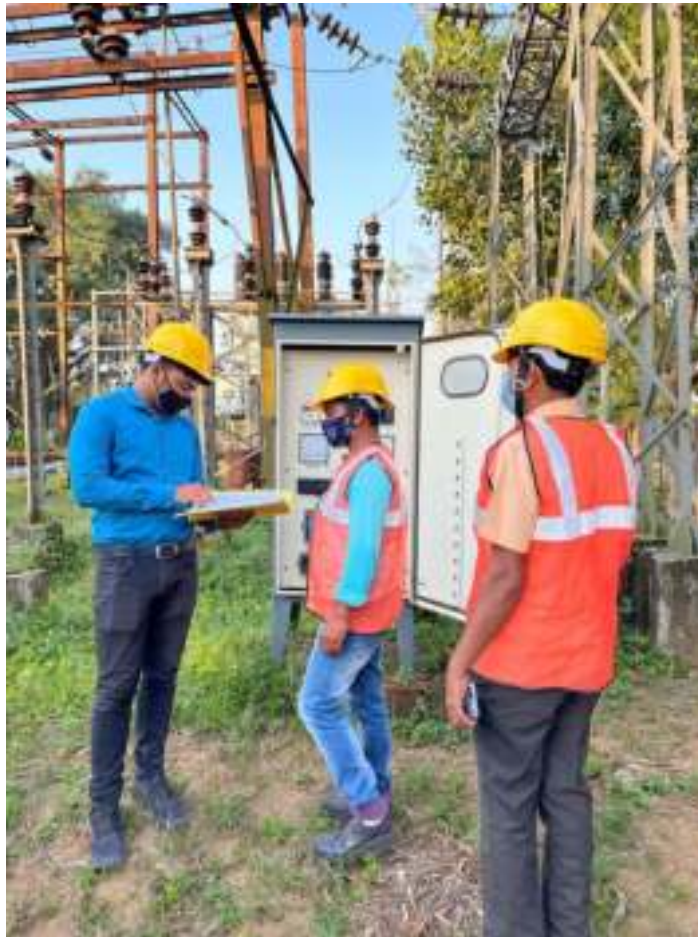
Visit to 33/11 kV PSS.
