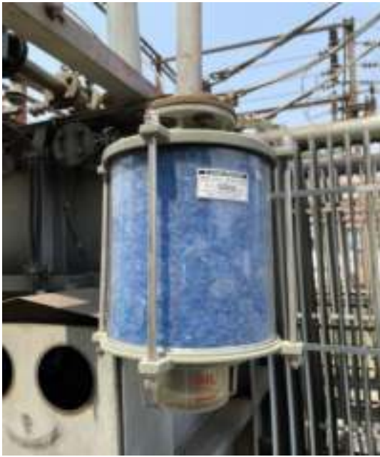
Silica Gel of transformer
