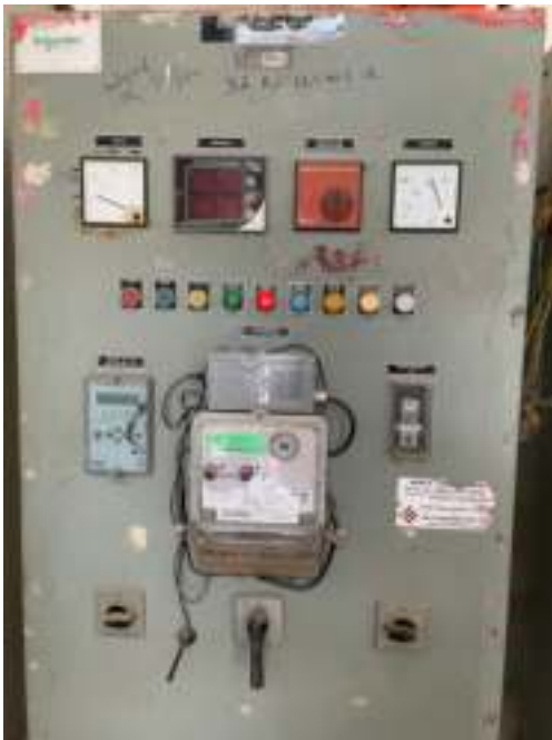
33 kV Control Panel
