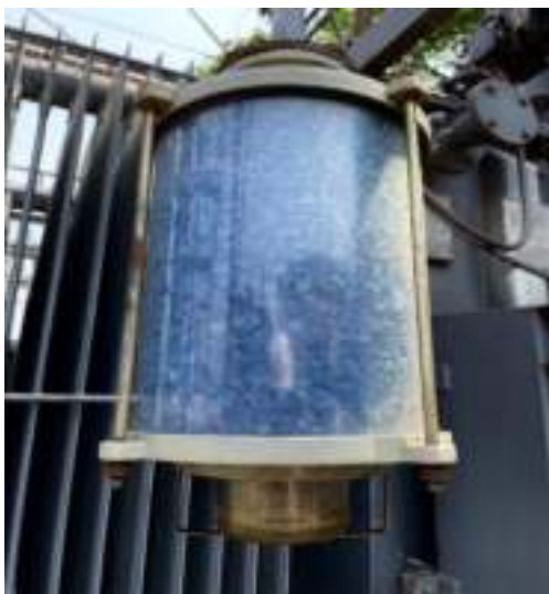
Silica Gel in Transformer
