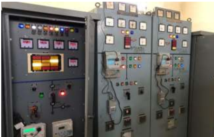
33kV and 11kV control panel
