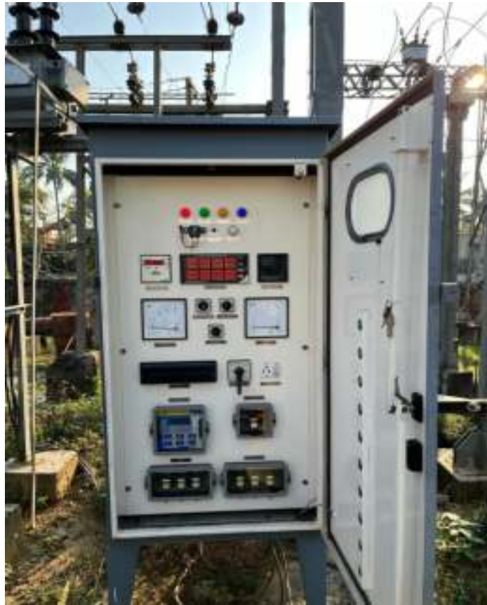
Jagannathpur feeder control panel
