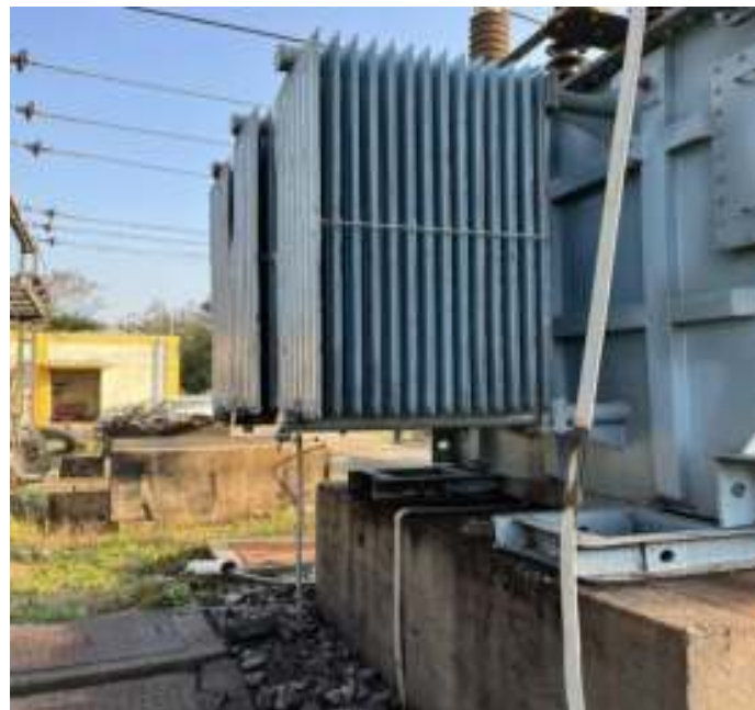
Mainda substation Power Transformer
