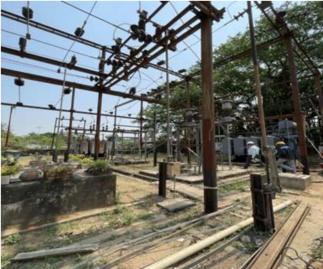
Physical Visit to Sovarampur 33/11 kV PSS
